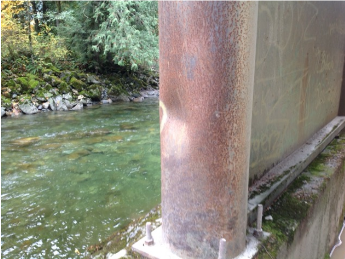
damage to upstream pier pipe column
