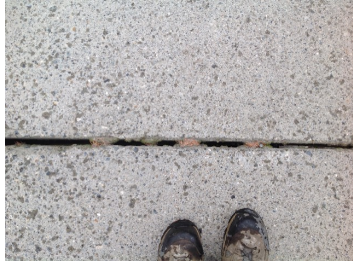
compression seal missing
