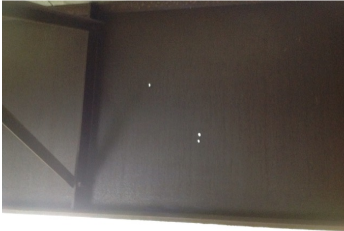
bullet holes through web of upstream girder
